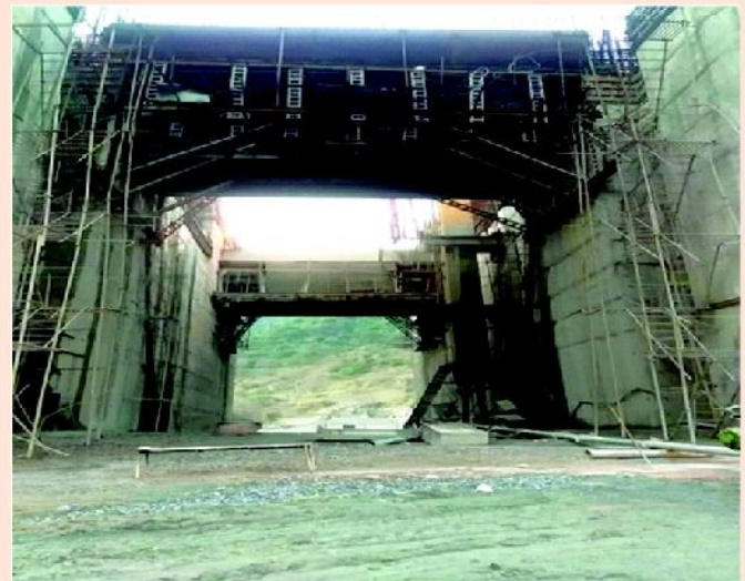
Orifice Radial Gate # 2
